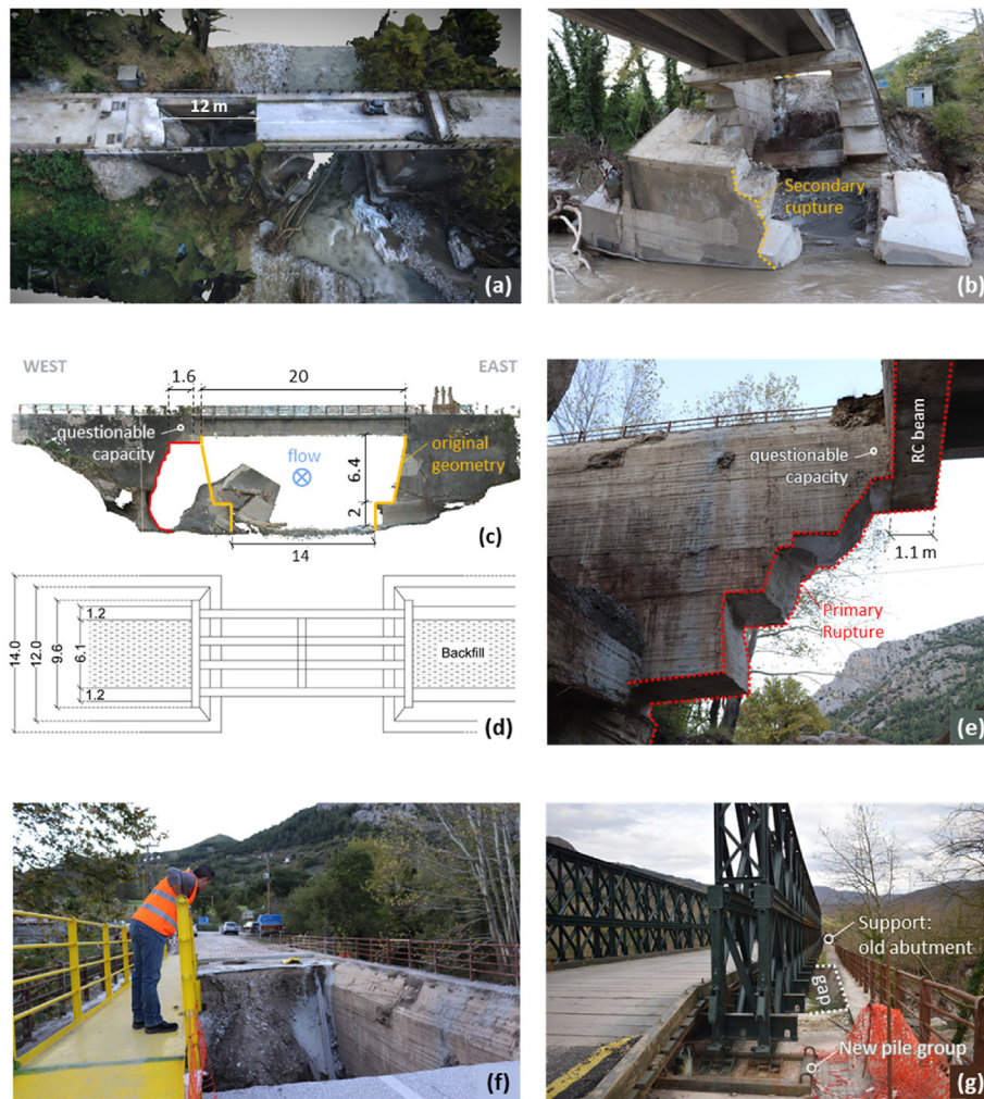
Fig. 4. Bridge 9: (a) 3D mesh model constructed using UAV images; (b) photo of the fractured unreinforced concrete abutment; (c) elevation and (d) plan view; (e) closer view of the failure pattern at the northern (downstream) wall; and (f) photo of the temporary emergency passage on 14 October 2020; and (g) the mitigation solution including the construction of a Bailey bridge on 28 November 2020.
